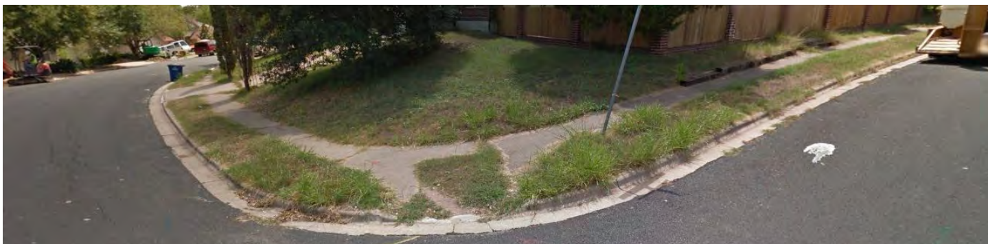
Sidewalk curb cut in disrepair at Lark Creek Drive and Gnarled Oak Cove in Austin
