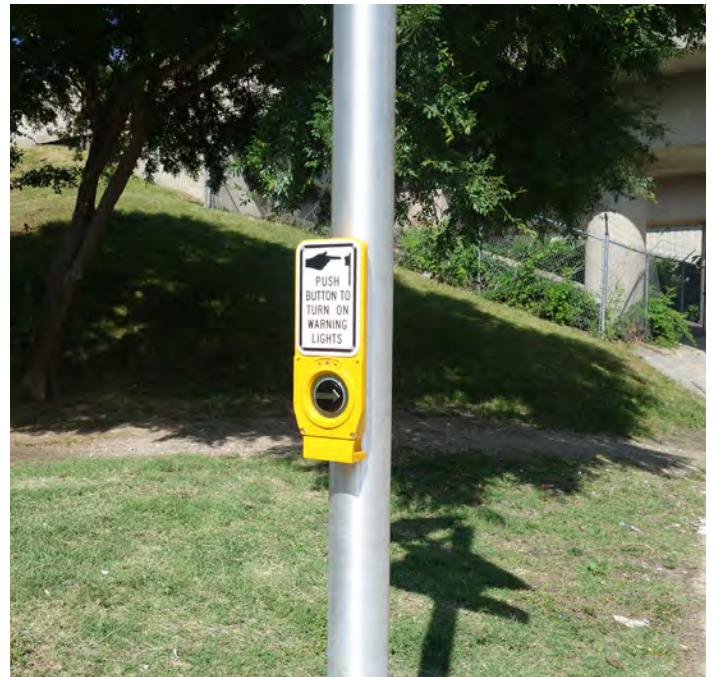
Electronic pedestrian push button at traffic signal
