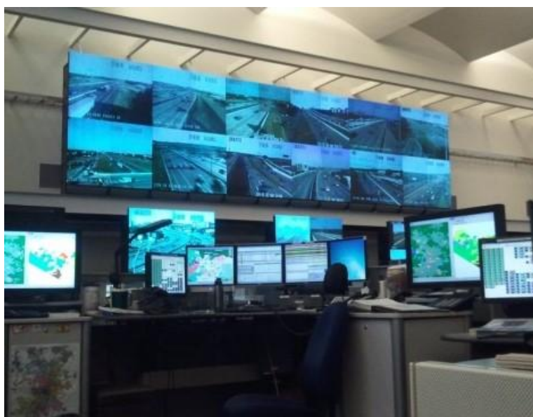
Figure 9 – Traffic management operators at CTECC use CCTV cameras, DMS and other transportation technologies to promote safety and mobility in the Region.
